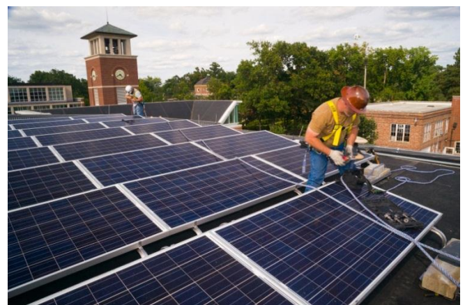
The solar panel arrays are part of a 20 year lease program, and the installations were done with no up-front cost to the University.
